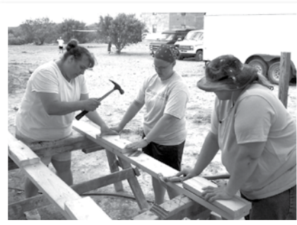
Amateur carpenters building bunk bed frames. Above, Matthew Rakestraw with three new buddies.
